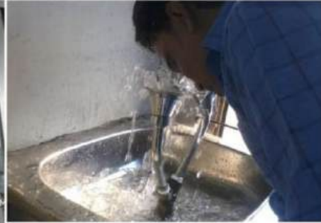
Eye wash Facility at Spot Removing Room
