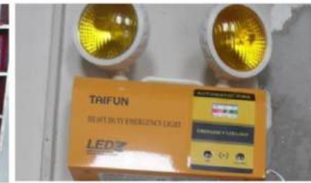
Emergency Fog Light in all Exit Point & Aisles of Production Floor
